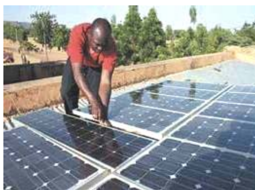
Figure 15: Solar panels on Roof top
